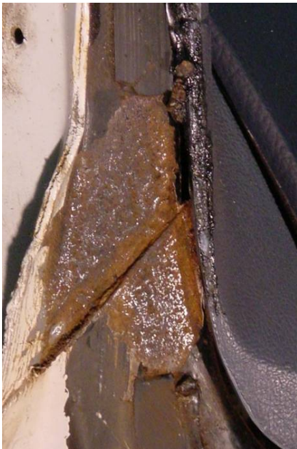
(Level 2 – 3 corrosion of pinchweld)
